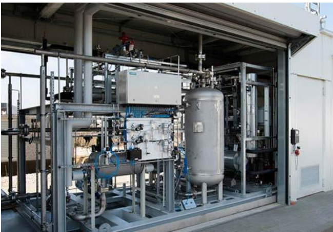
Figure 1: Sample image of McPhy Electrolyzer plant
