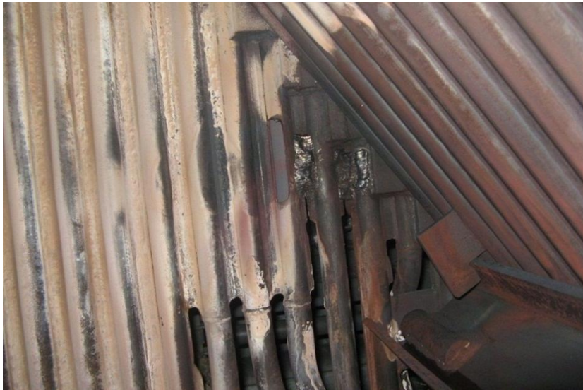
Figure 1: An example of typical boiler tube failure locations
